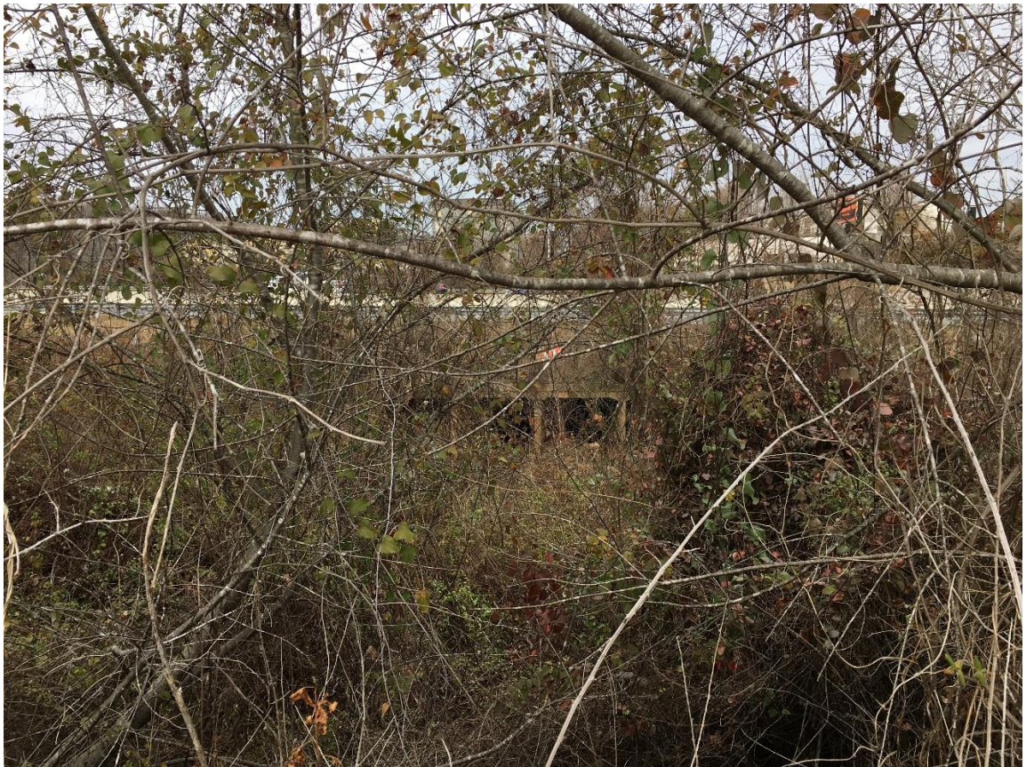
Looking upstream at I-85 box culverts at Rocky Creek from Honbarrier Drive.
