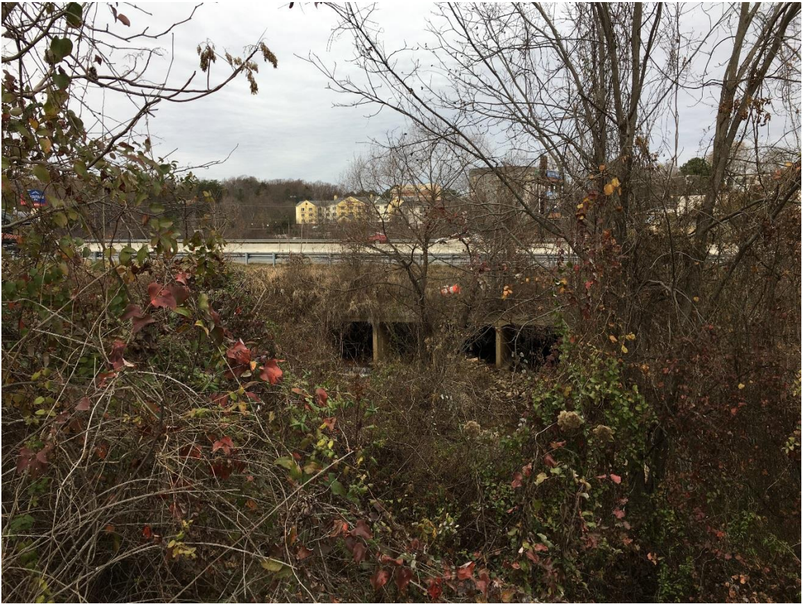
Looking upstream at I-85 box culverts at Rocky Creek from Honbarrier Drive.
