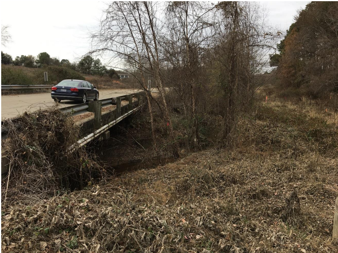
Looking southwest at the upstream face of the Honbarrier Drive bridge over Rocky Creek.
